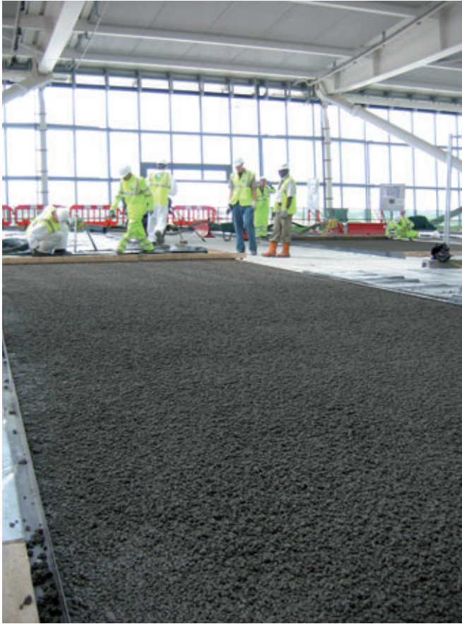
Fig. 2: Constructing the lightweight LYTAG no fines base coat screed for Heathrow's new Terminal 5, UK
